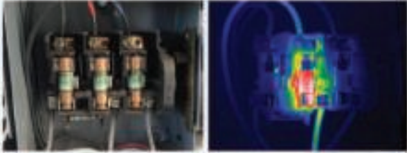
FAULTY / CORRODED FUSES
