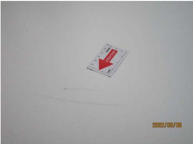
01 defect-minor-scratch mark (3.5cm) on unit
